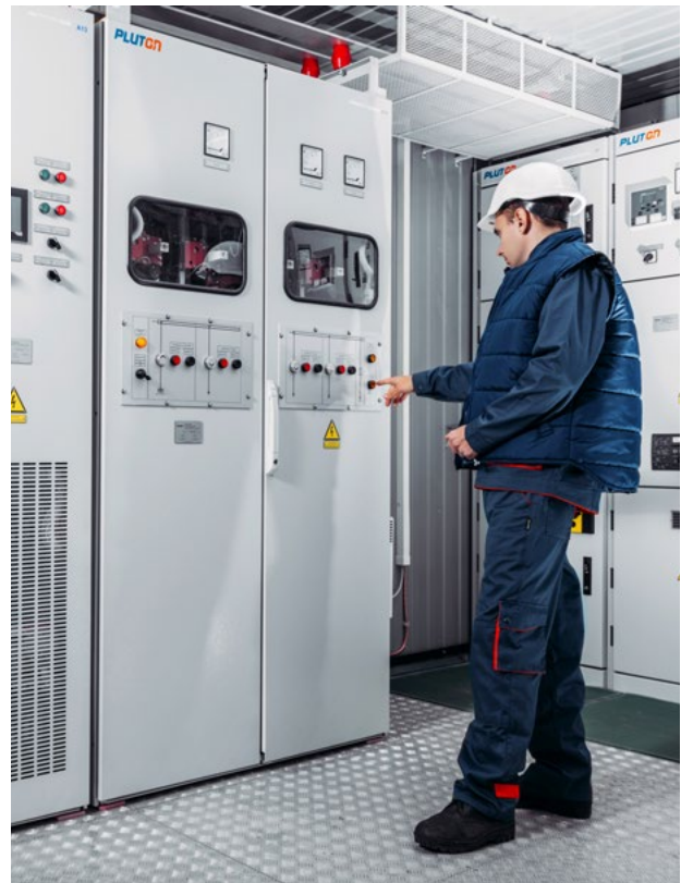
▲ Negative busbar switchgear
