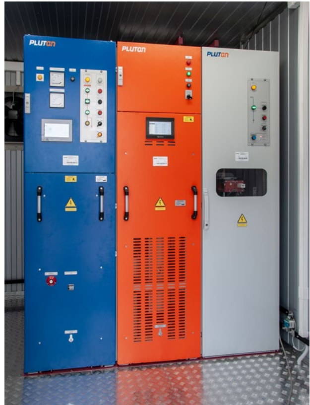
▲ Negative busbar switchgear (on the right), withdrawable rectifier (in the middle) DC switchgear (on the left)
