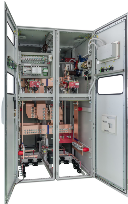
▲ Negative Switchgear for railway
